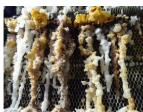
Halite scaling on the borehole heat exchangers
