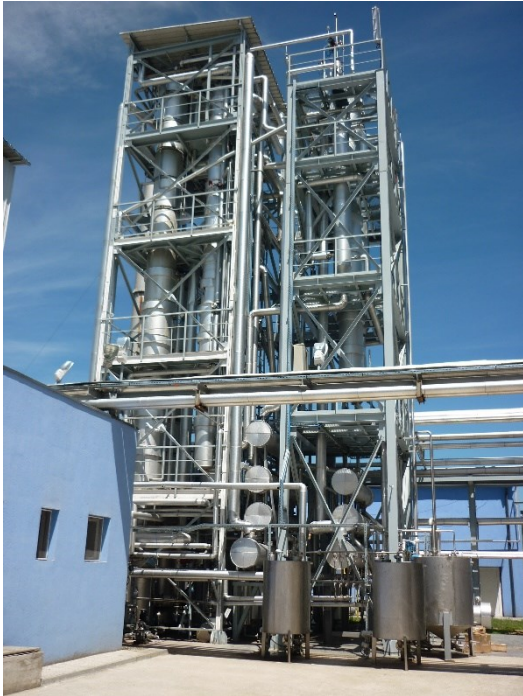
Fig. 17. Photograph of a rectification plant for ethanol production with productivity of 20000 litres/24h consisting of five columns with Holpack packing
