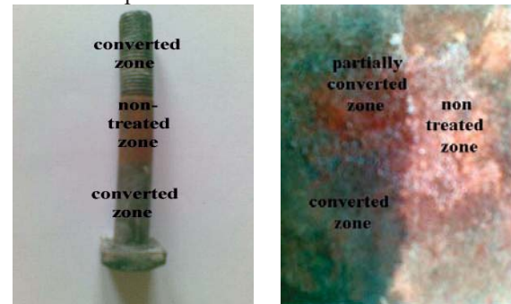
Fig. 4. Images of rusted stud (left) and iron plate (right) after treatment with LR-3.
