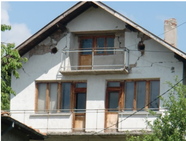
Fig. 1. Damages caused by the 2012 M_w 5.6 earthquake.
