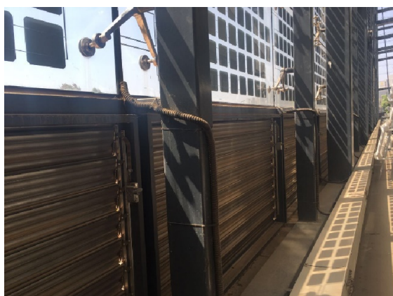
Fig.6. The ventilation blinds at the top and bottom of the PV curtain wall
