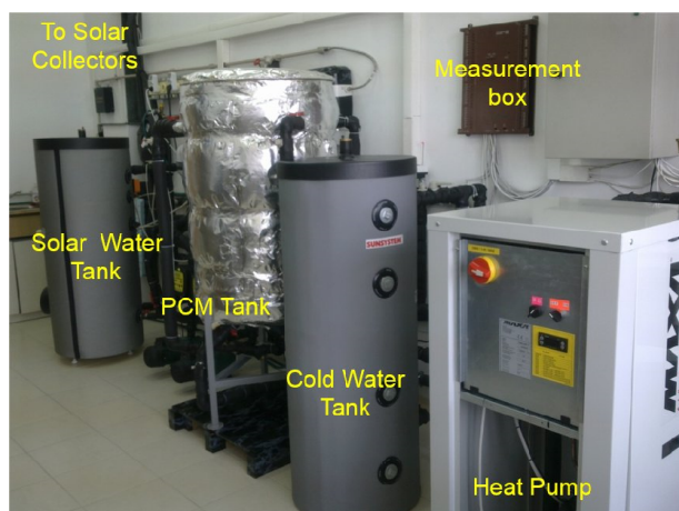
Fig.14. Interior laboratory view of the hybrid installation
