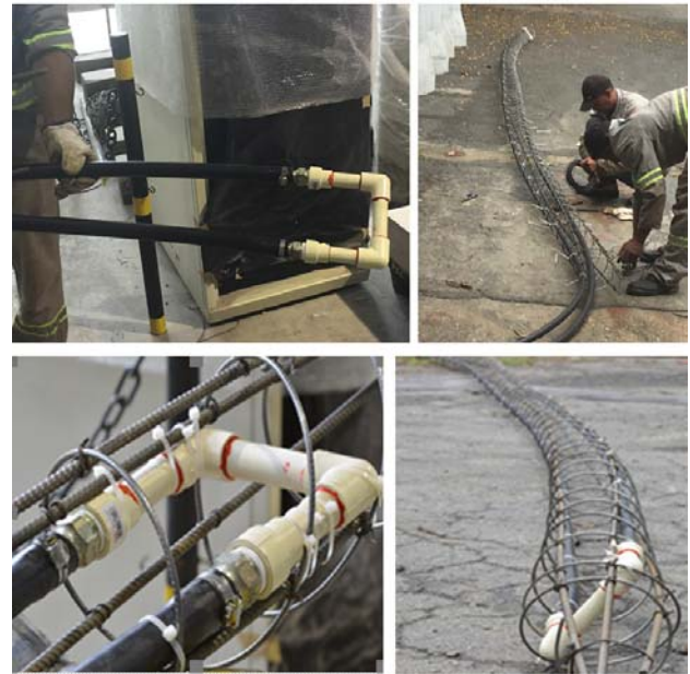
Fig.3. Installation of the U-shaped exchanger tubes in the reinforcement cage of the micropile
