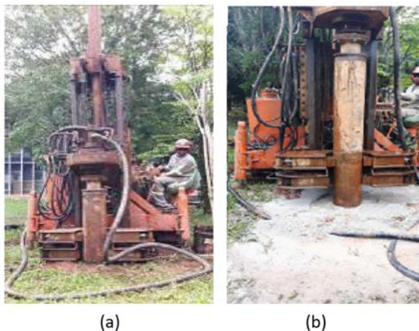
Fig.2. Construction of the energy pile: a) hydraulic drilling rig, and b) drilling process
