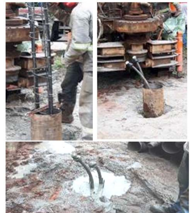
Fig.4. Construction of the energy pile: installation of the reinforcement cage with a U-shaped heat exchanger tube
