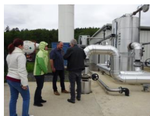
Reinjection borehole and hydrothermal power plant
