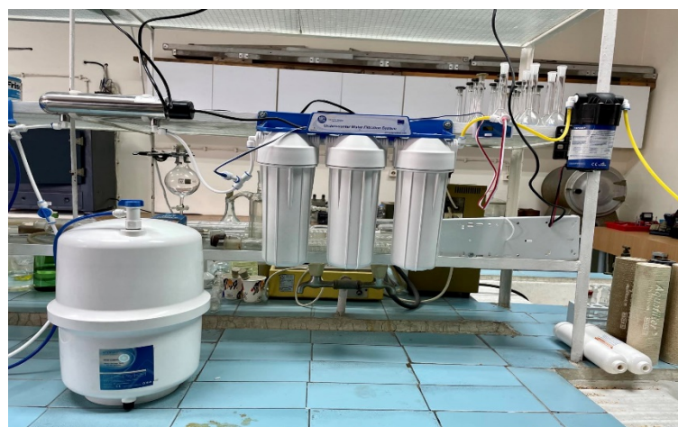
Fig. 3. Spring water purification system with filtration and UV – disinfection (Module 2).
